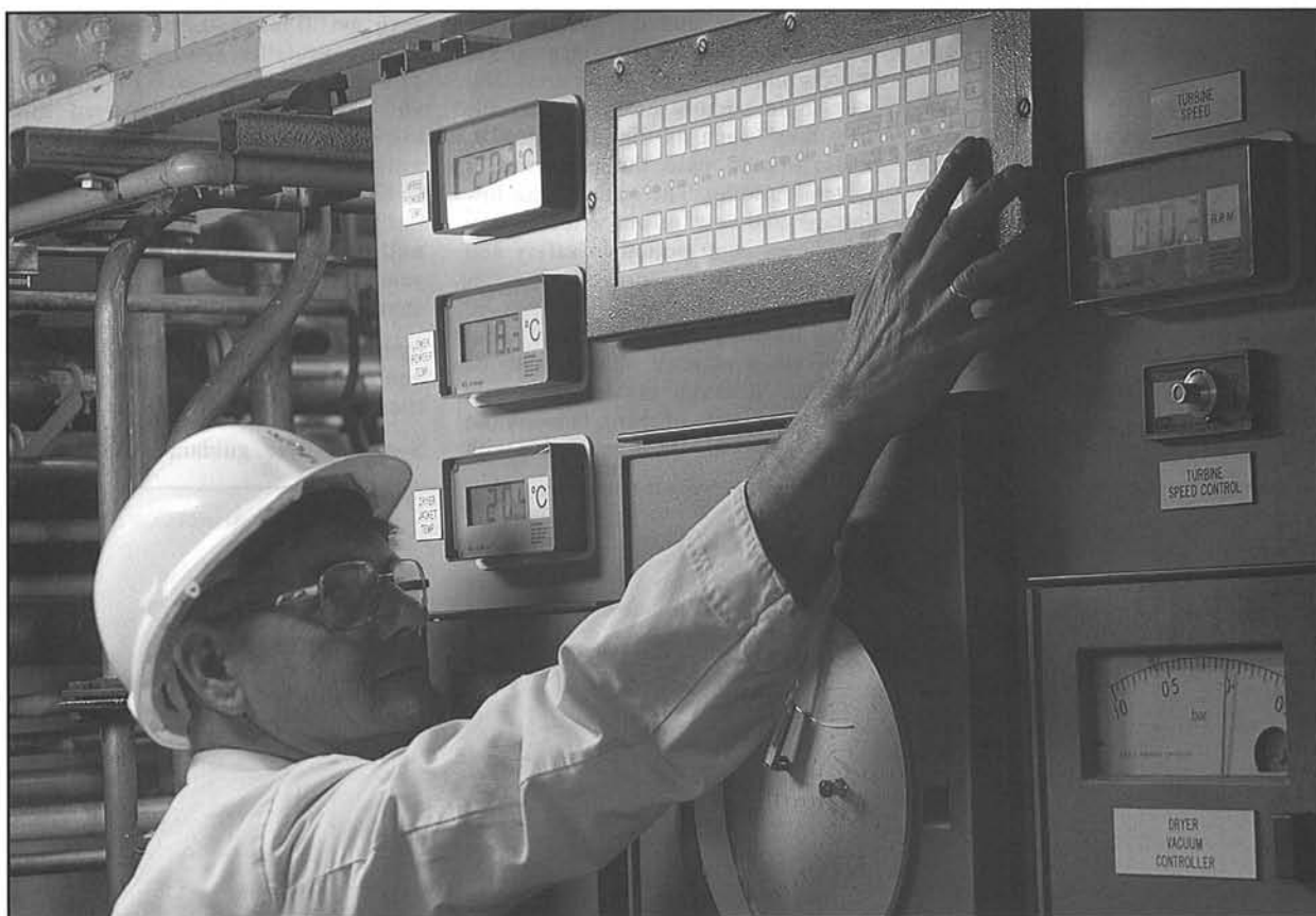
Fig. 8. Plant mounted intrinsically safe indicators and annunciators
